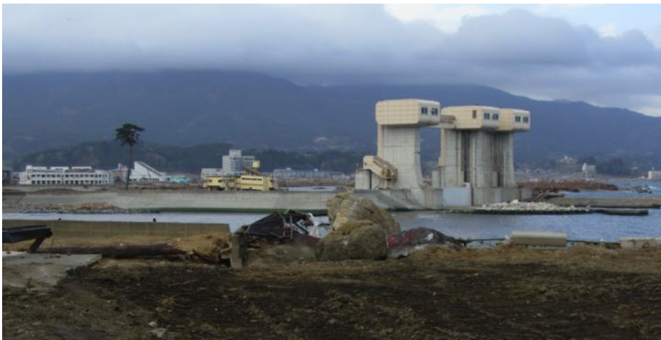
Damaged floodgate control system at Rikuzentakata. A number of firemen perished while attempting to close the gates. The lone surviving pine tree is to the left.
